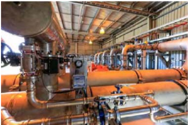
Monreagh Pump Station - inside view
