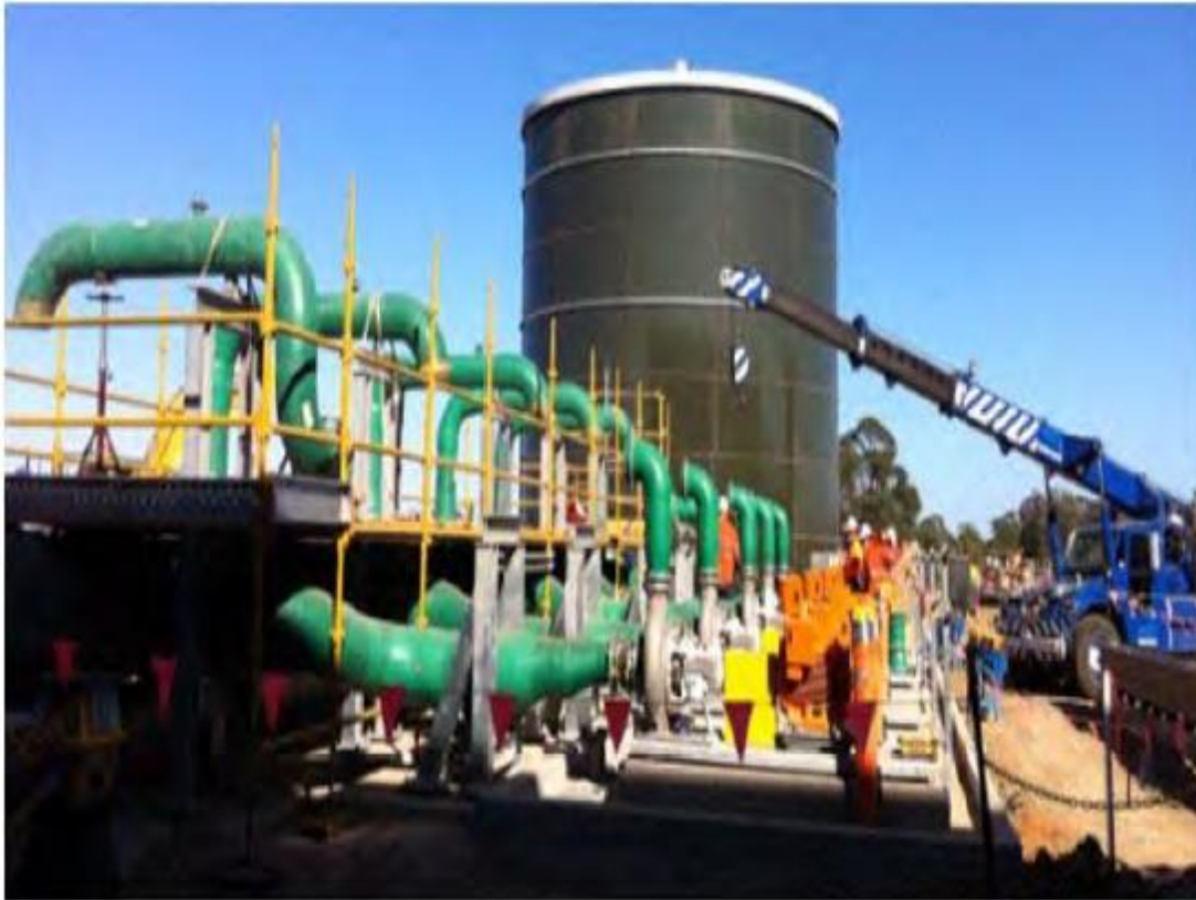
Water Treatment Facility - Condabri Central
