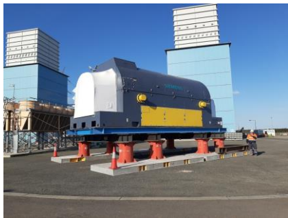
New stator on-site at Mortlake
