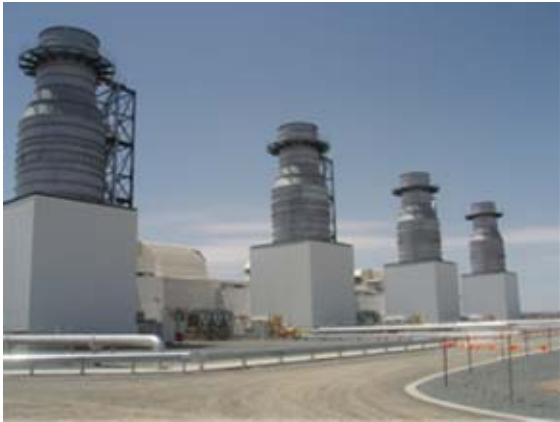
All 4 completed Uranquinty PS turbines
