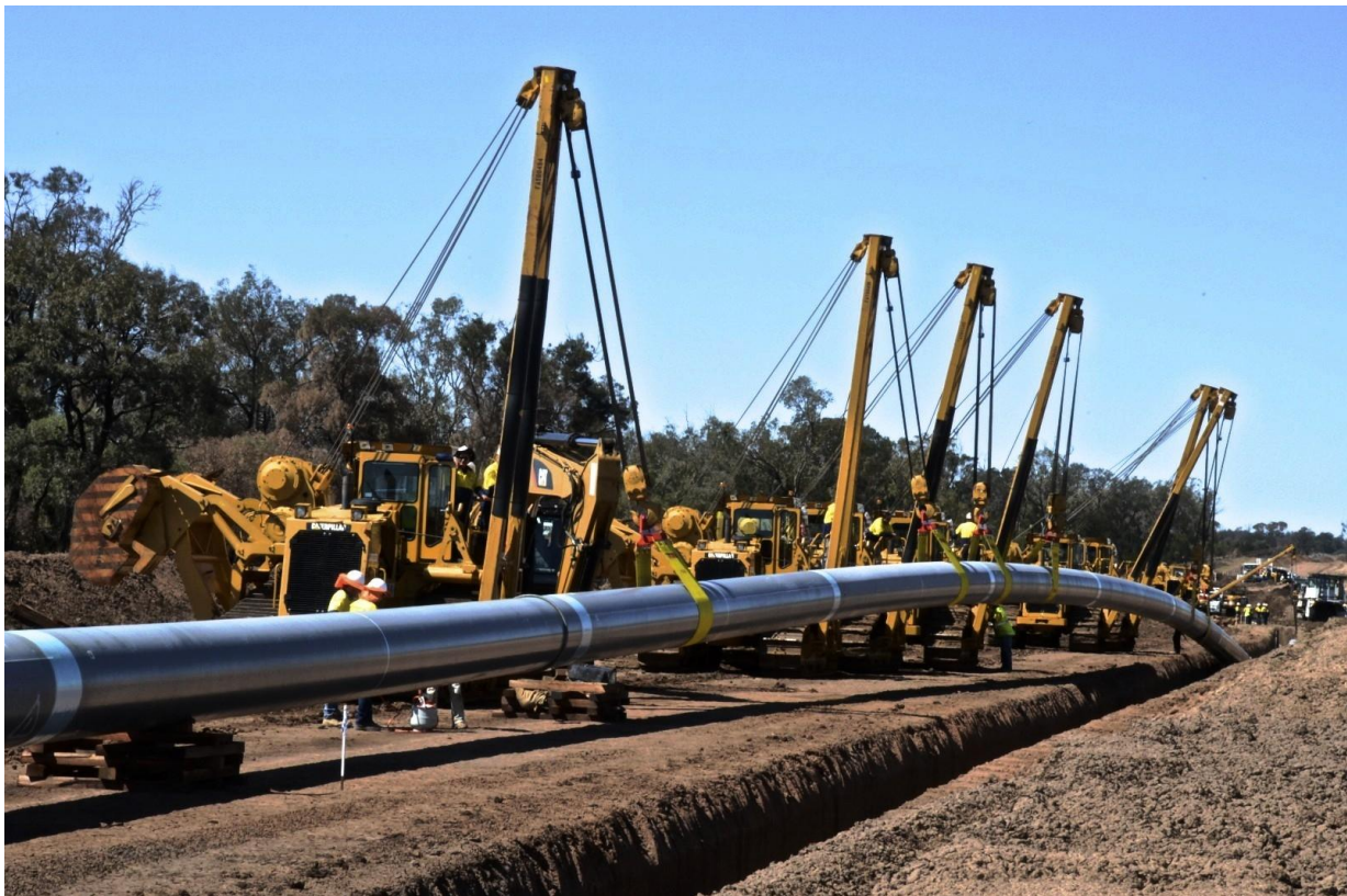
The first of more than 530km of pipe being laid, south of Miles, October 2012
