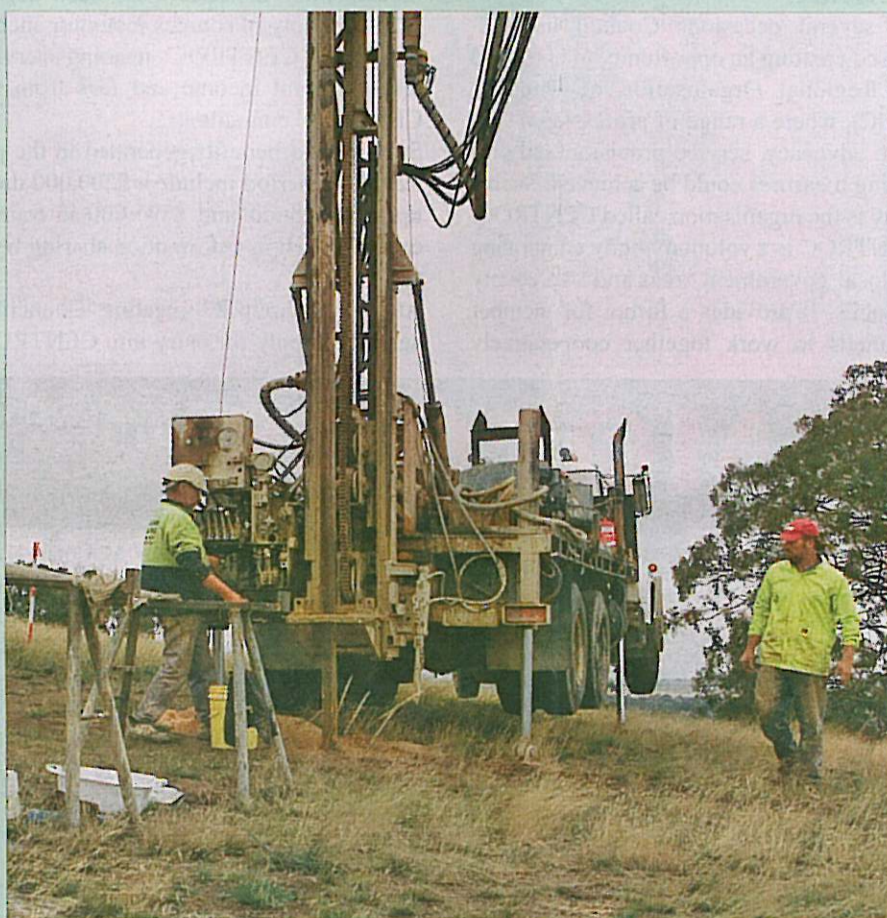
In February 2008, core samples were taken to establish geotechnical conditions for turbine foundations.
