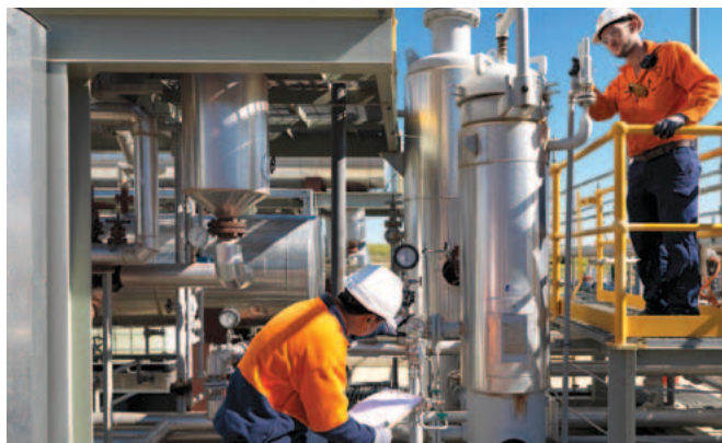
Origin employees at the Spring Gully Gas Plant
