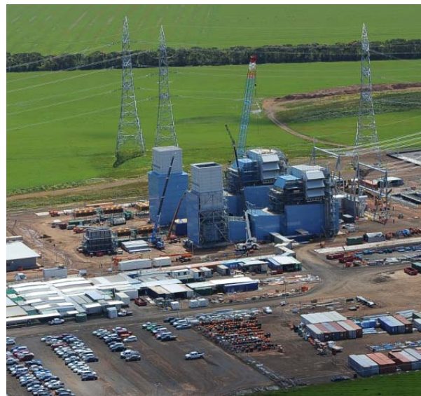
Aerial shot of Mortlake Power Station
