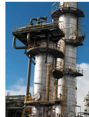
Otway gas processing plant
