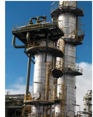
Otway gas processing plant
