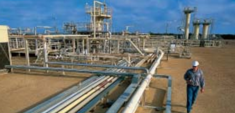
Beharra Springs Processing Plant, Perth Basin, WA.
