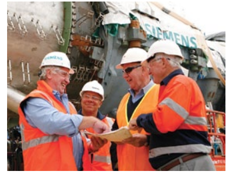
Origin and Lend Lease Infrastructure Services site managers discuss the onsite turbine construction with Siemens engineers.
