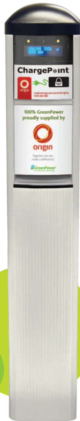
An Origin ChargePoint charging station
