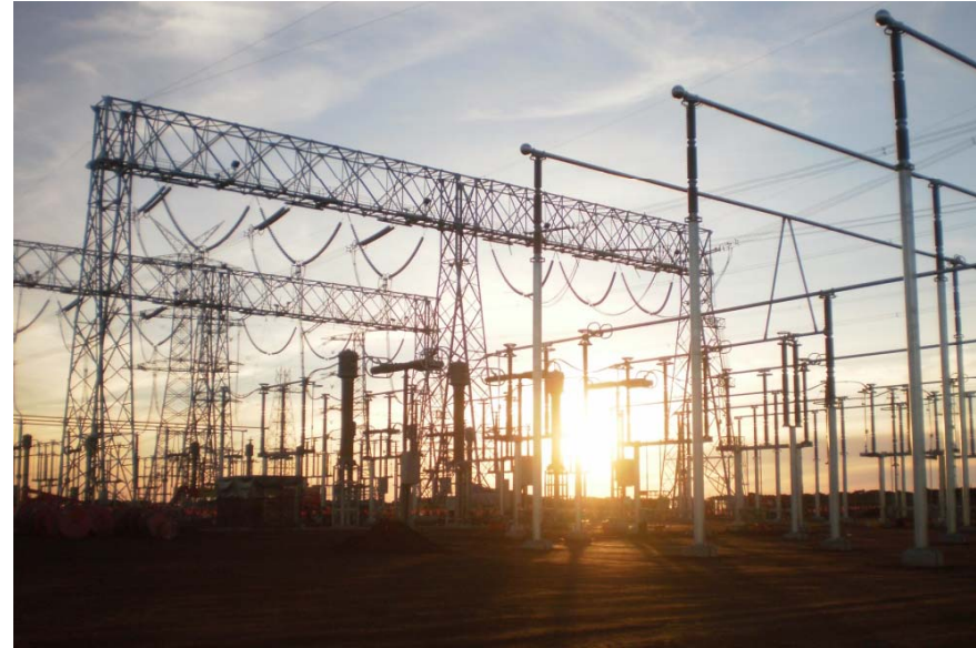
Mortlake Power Station switchyard
